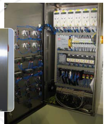
ABOVE: Control panel by JWCI.
