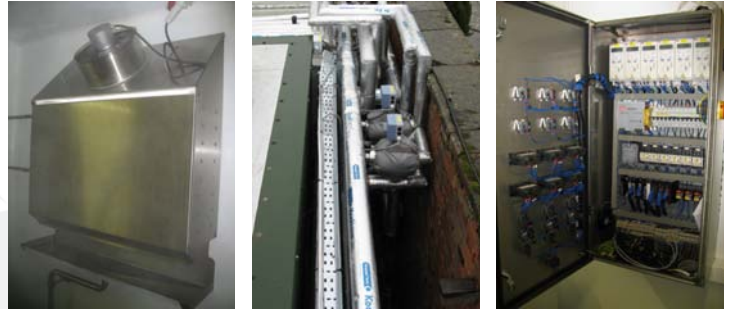
ABOVE: An additional four coolers for the maturation stores designed, manufactured and installed by JWCI with all valves and control panels.
