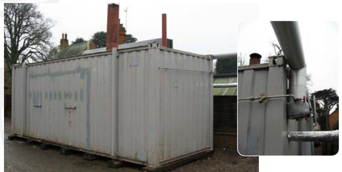
ABOVE: Containerized Boiler Unit manufactured off site and installed to run alongside the original small boiler.
